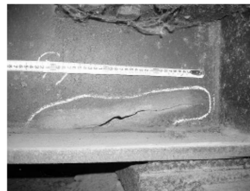
Crack due to fatigue
